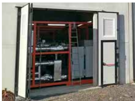
Città della Pieve (PG, Italy) - Power generation from biomass-fueled boiler (pruning residues)
