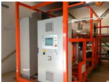
Rovato (BS, Italy) - Power generation from biomass-fueled boiler (end-of-life pallets)
