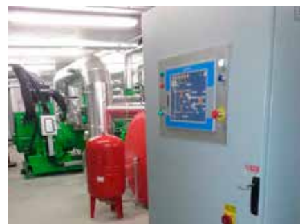
Morgex (Aosta) - Heat recovery from cooling jackets and exhausts of vegetable oil-fueled engines
