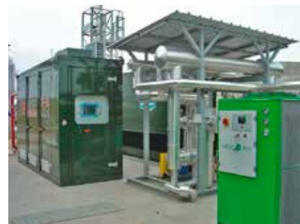
Portogruaro (Venice) - Heat recovery from cooling jackets and exhaust gases of biogas-fueled engines
