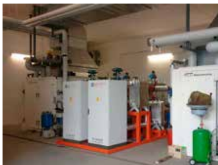
Renon (Bozen) - Heat recovery from cooling jackets and exhausts of vegetable oil-fueled engines
