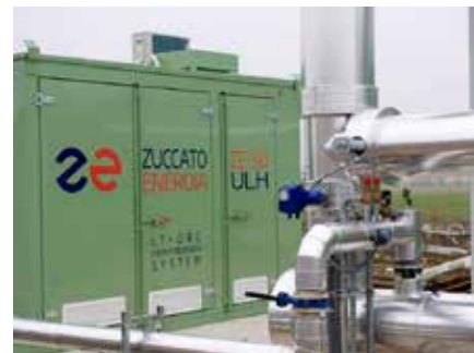
Borgoforte (Mantua) - Heat recovery from cooling jackets and exhausts of biogas-fueled engines
