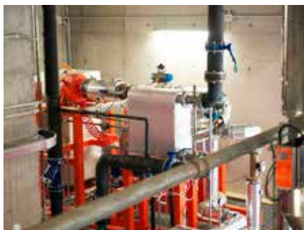
Mestre (Venice) - Heat recovery from biomass boiler and hot air turbines
