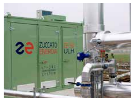
Borgoforte (MN, Italy) - Heat recovery from jackets and fumes of biogas-fueled gensets
