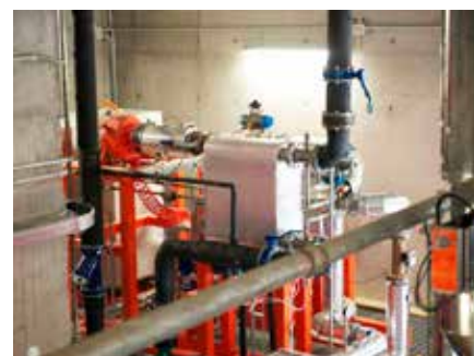
Mestre (VE, Italy) - Heat recovery from biomass-fueled boilers and hot-air turbines
