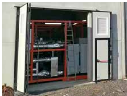
Città della Pieve (PG, Italy) - Power generation from biomass-fueled boiler (pruning residues)
