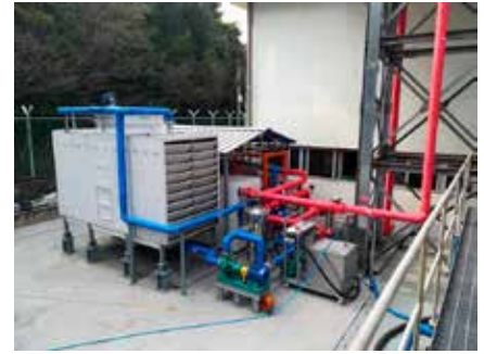
Heuksan (South Korea) - Heat recovery from thermoelectric power station (heavy oil gensets)
