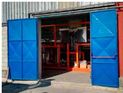
Castrovillari (CS, Italy) Power generation from biomass-fueled boiler (pruning residues)
