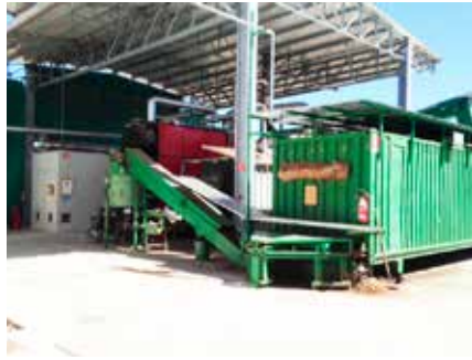
Sommalombardo (VA, Italy) - Power generation from biomass-fueled boiler (sawmill residues)
