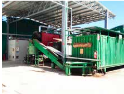
Sommalombardo (VA, Italy) - Power generation from biomass-fueled boiler (sawmill residues)
