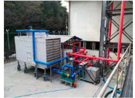
Heuksan (South Korea) - Heat recovery from thermoelectric power station (heavy oil gensets)
