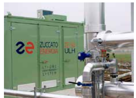
Borgoforte (MN, Italy) - Heat recovery from jackets and fumes of biogas-fueled gensets
