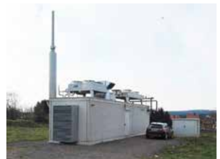
Benneckestein (Germany) - Heat recovery from jackets and fumes of biogas-fueled gensets
